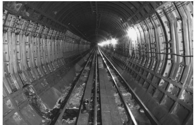
Old Street: acid attack on tunnel lining ( https://www.londonreconnections.com/2013/a-cid-works/ )
